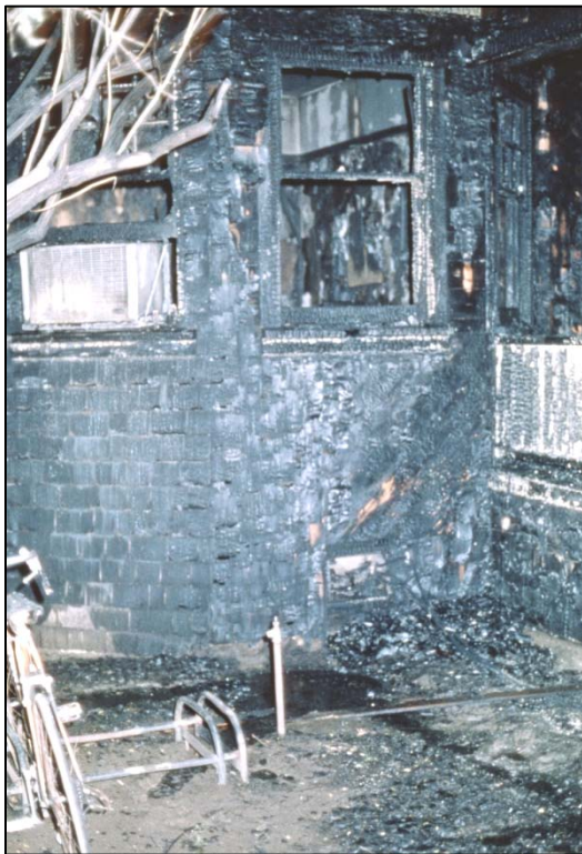
Photograph the exterior of the building to show the extent of fire damage and locations of doors and windows.
